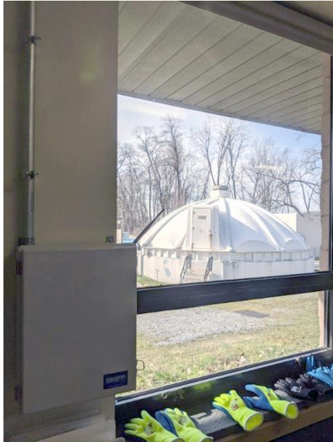
PDW Base Station with Remote, External-to-Building Antenna
