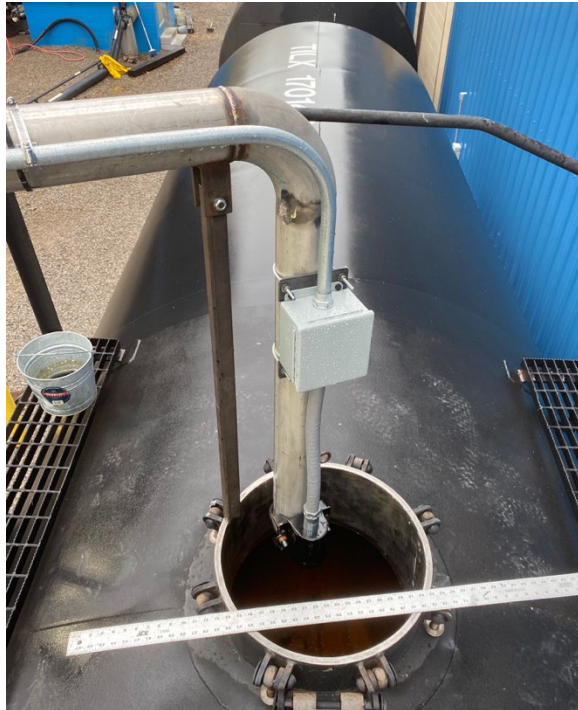
Radar Level Transmitter on Swivel Loading arm
