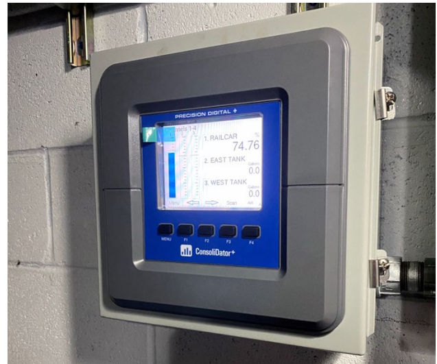
PD9000 ConsoliDator+ in a PDA2909 NEMA 4 Wall/Field Mount Enclosure (Note: Picture Taken Before Setup Complete)
