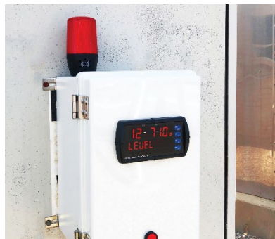
Meter in Enclosure with Light / Horn on Side of Tank
