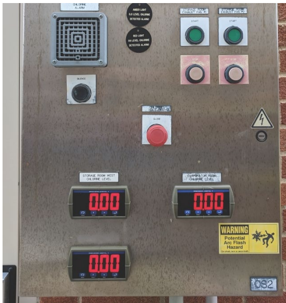
Chlorine Leak Detection
