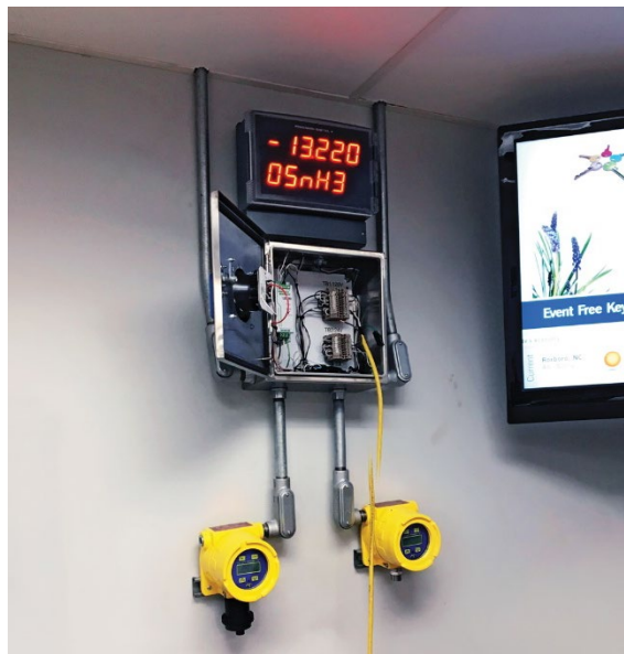
Displaying Outside Ammonia
