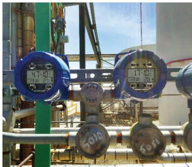
Hazardous Area Level Display in Tank Farm
