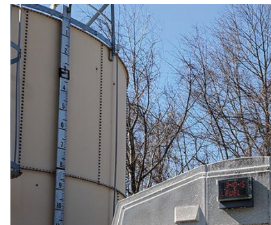
Display Tank Height in Feet & Inches Outdoors Next to Tank
