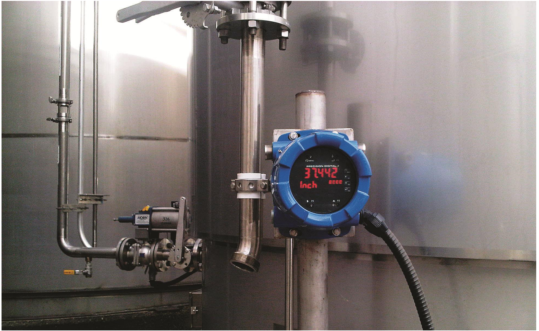
PD8-6000 - Oil Tank Level Indication
