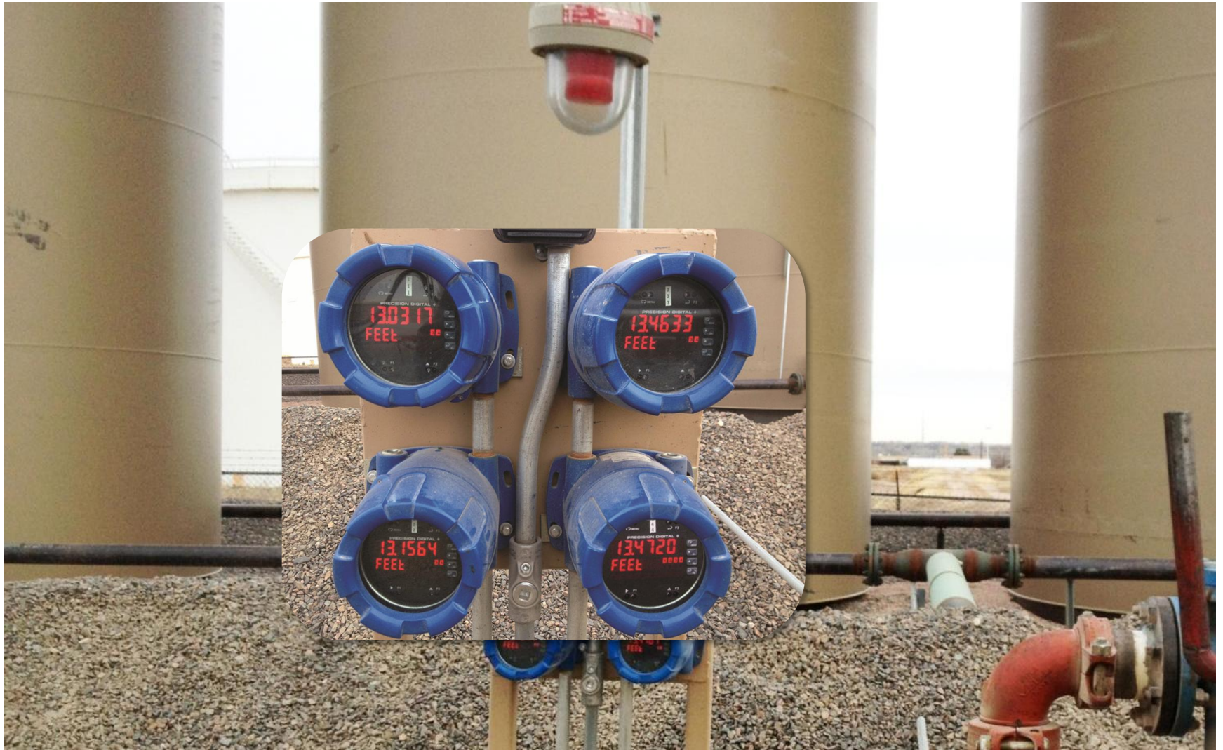
PD8-6000 – Crude Oil Holding Tank Level Monitoring
