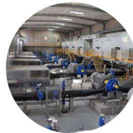
LIFT & PUMP STATION CONTROL
