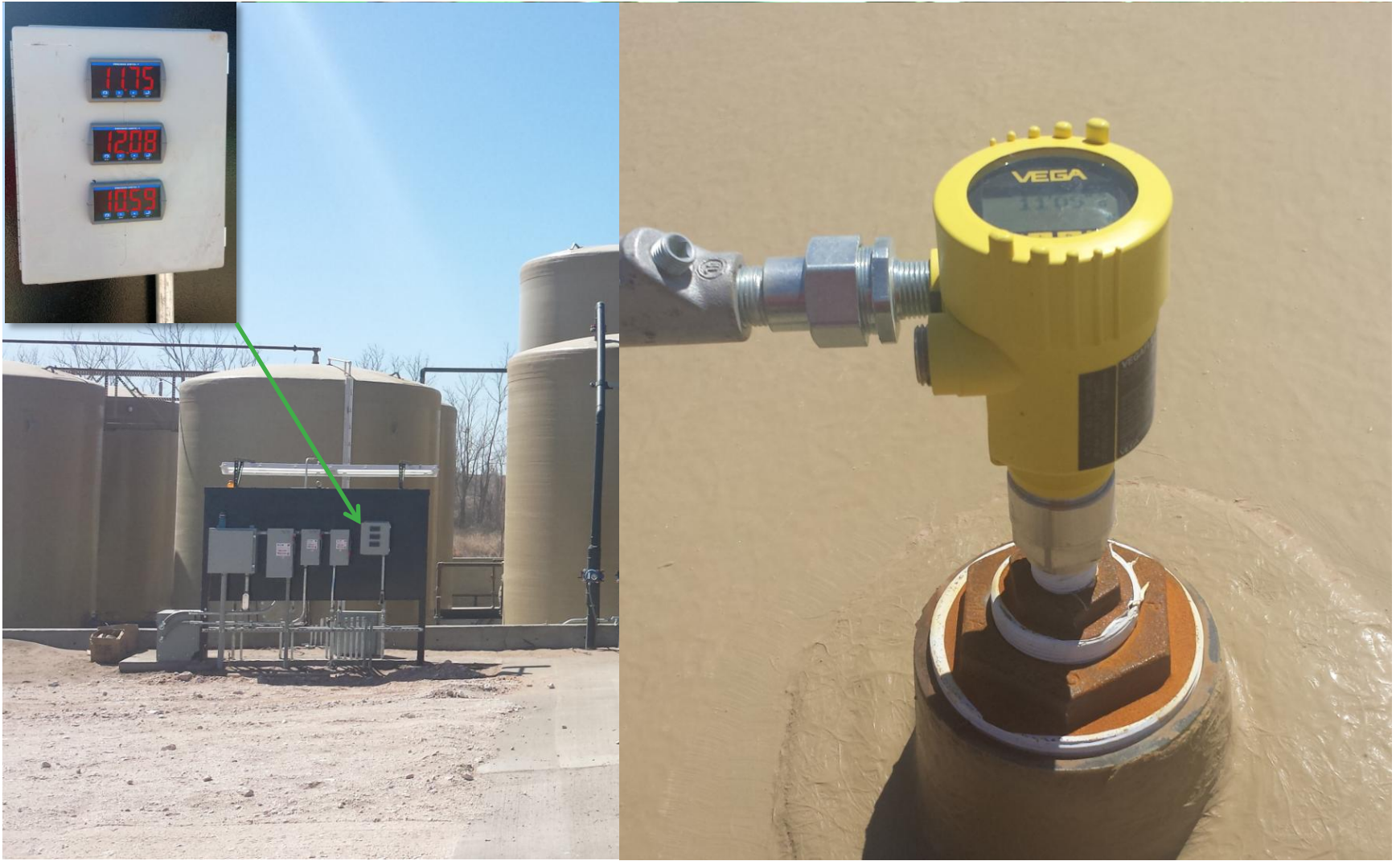
PD765 X2 – Salt Water Tank Level at Truck Loading Stations
