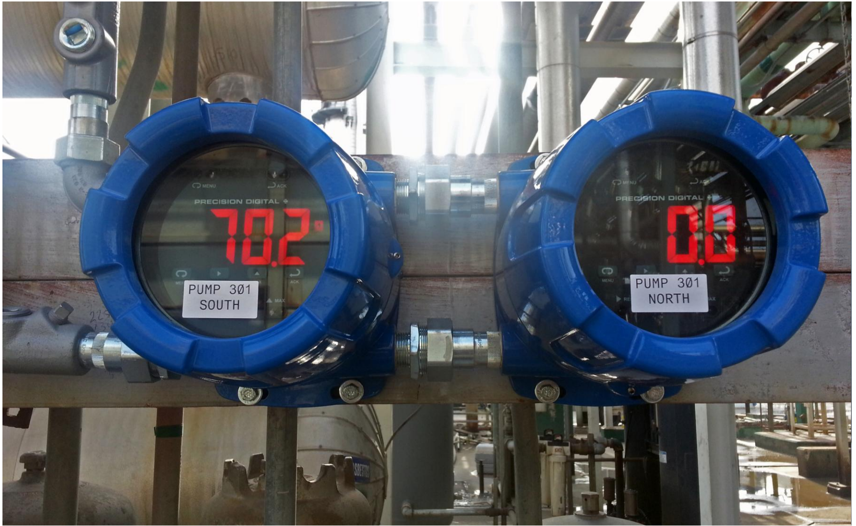
PD8-765 – Level Indication & Pump Control at Oil Refinery
