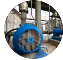
Pump Alternation Control
