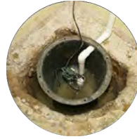
Sump Level Monitoring
