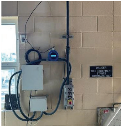
PDW90-FN Connected to 4-20 mA Sensor Inside the Building
