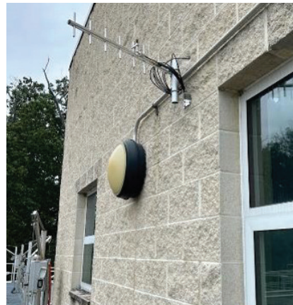
PDA3900 Yagi Antenna Mounted Outside the Building
