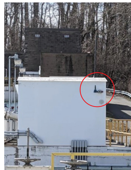
PDW90 Field Unit Installation at Aeration Basin Blowers
