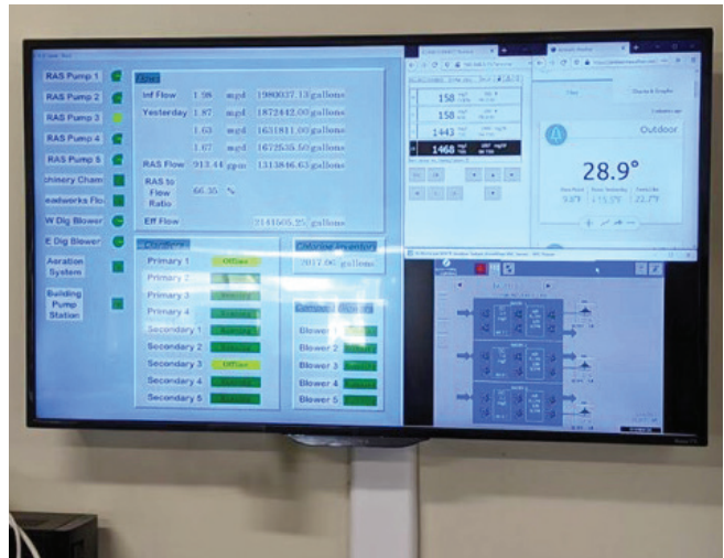
4-20 mA and Digital I/O go to the SCADA system
