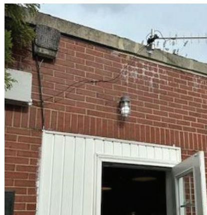
PDA3900 Yagi Antenna Mounted Outside the Building
