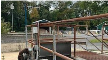
Yagi Antenna connected to the PDW90 Base Station
