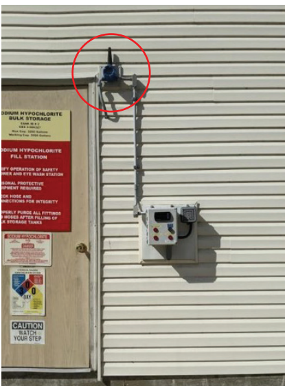
PDW90 Field Unit Installation at Storage Building
