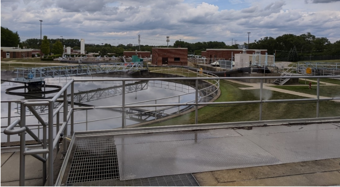
Wastewater Treatment Facility
