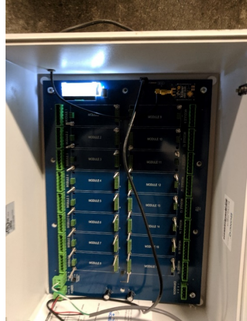
Inside the Base Station, No I/O Cards are Needed as all Readings were Modbus
