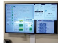
4-20 mA and Digital I/O go to the SCADA system
