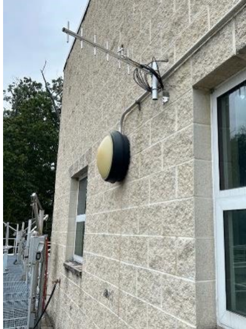
PDA3900 Yagi Antenna Mounted Outside the Building
