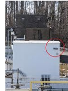
PDW90 Field Unit Installation at Aeration Basin Blowers
