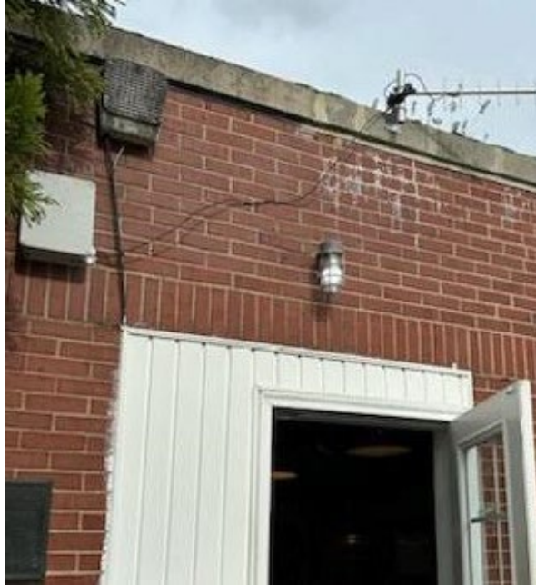
PDA3900 Yagi Antenna Mounted Outside the Building
