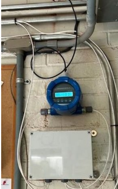
PDW90-FN Connected to 4-20 mA Sensor Inside the Building
