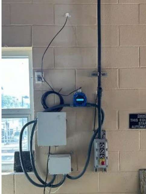
PDW90-FN Connected to 4-20 mA Sensor Inside the Building
