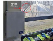
PDW90 Base Station with Attached Antenna Inside Building
