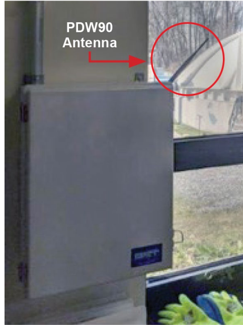
PDW90 Base Station with Attached Antenna Inside Building
